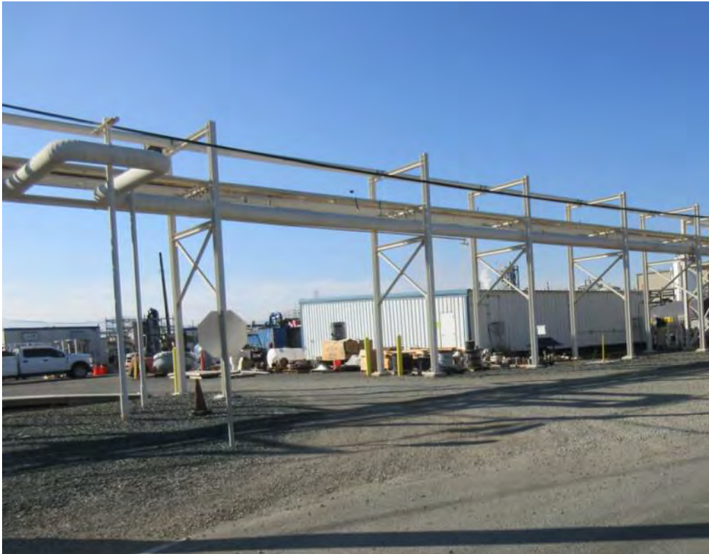
Existing Pipe Rack along 3 rd -Street (New chlorine line will be supported on upper level of this lightly loaded pipe rack)
