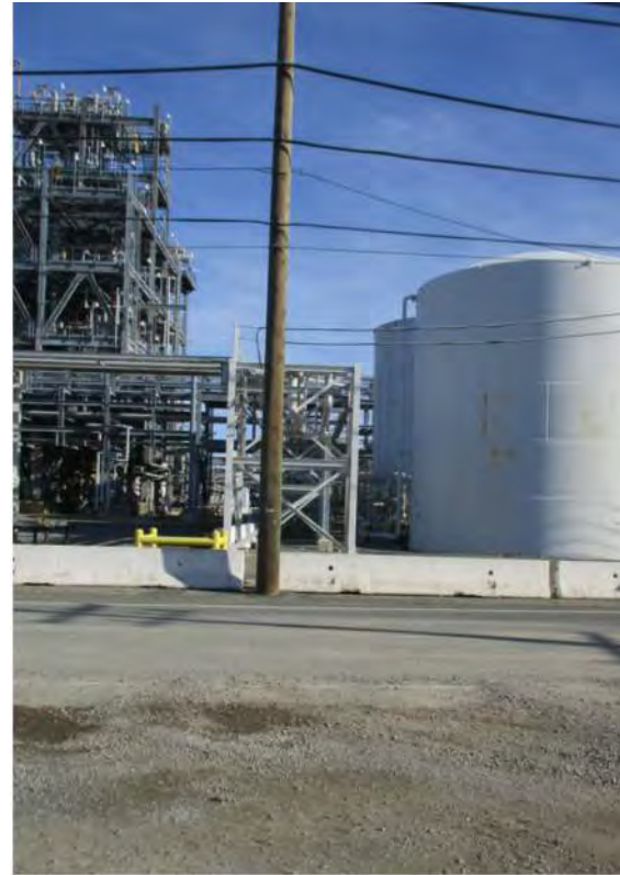
End of Existing N-S Pipe Rack to Douglas Products (Looking North) (New chlorine line will be supported on upper level of this lightly loaded pipe rack. New N-S bridge over 3 rd Street will be slightly east of the existing pipe rack)
