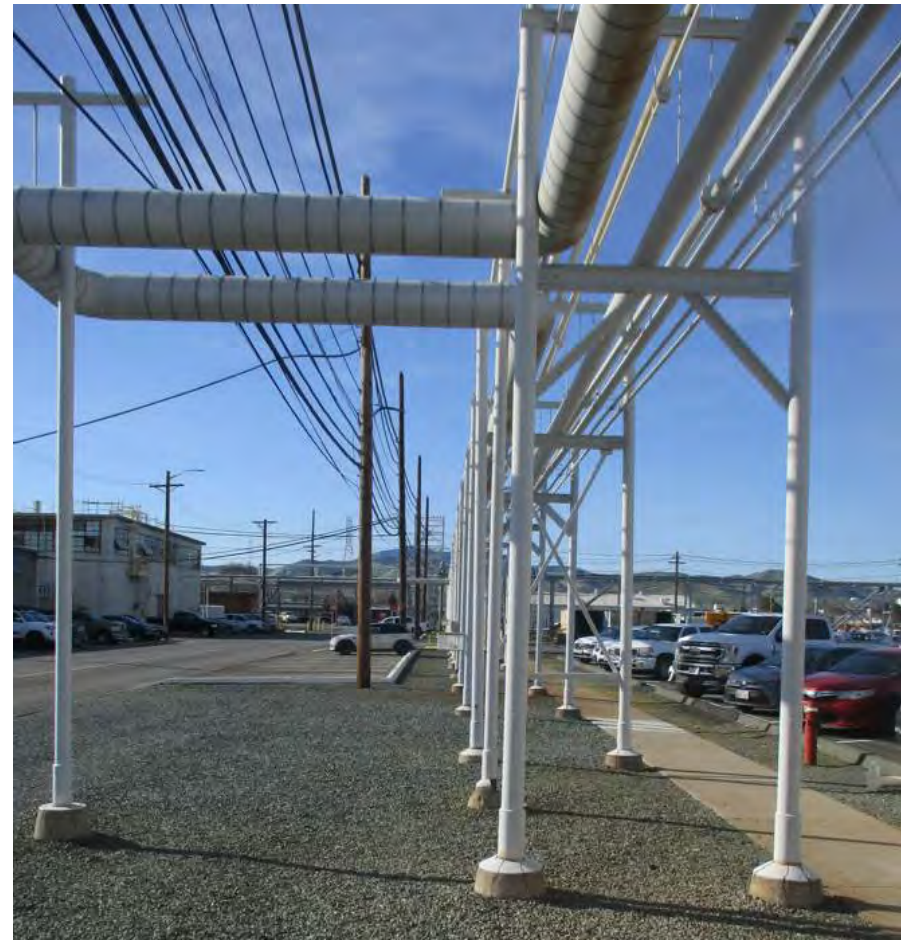
View Along E-Street from Building 344 (New supports will be just in front of existing pipe rack along E-Street to tie-in location)
