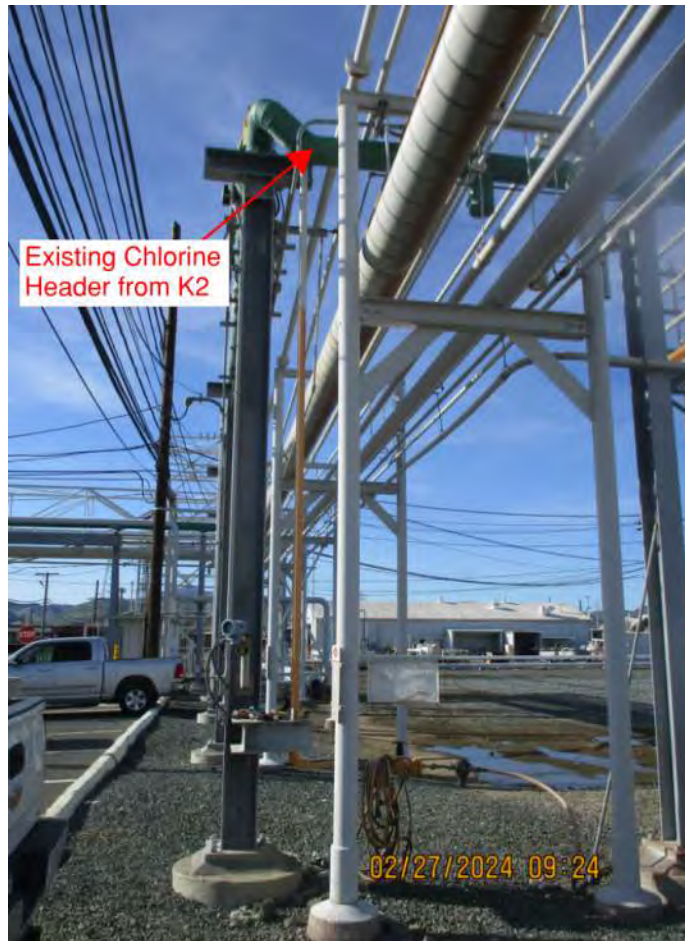
Tie-in Location (Looking South) (Elevation of new piping along E-Street will match existing)
